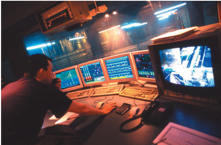
Figure 55: Inside the IT-Cockpit: One person at a time is able to monitor and control all the operations.
